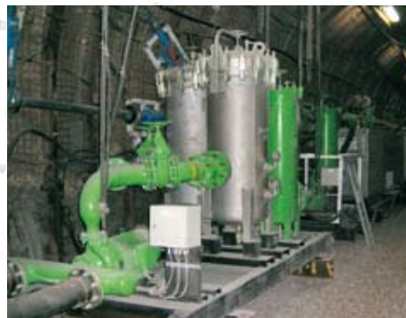
Pump Station for supplying HFA.
